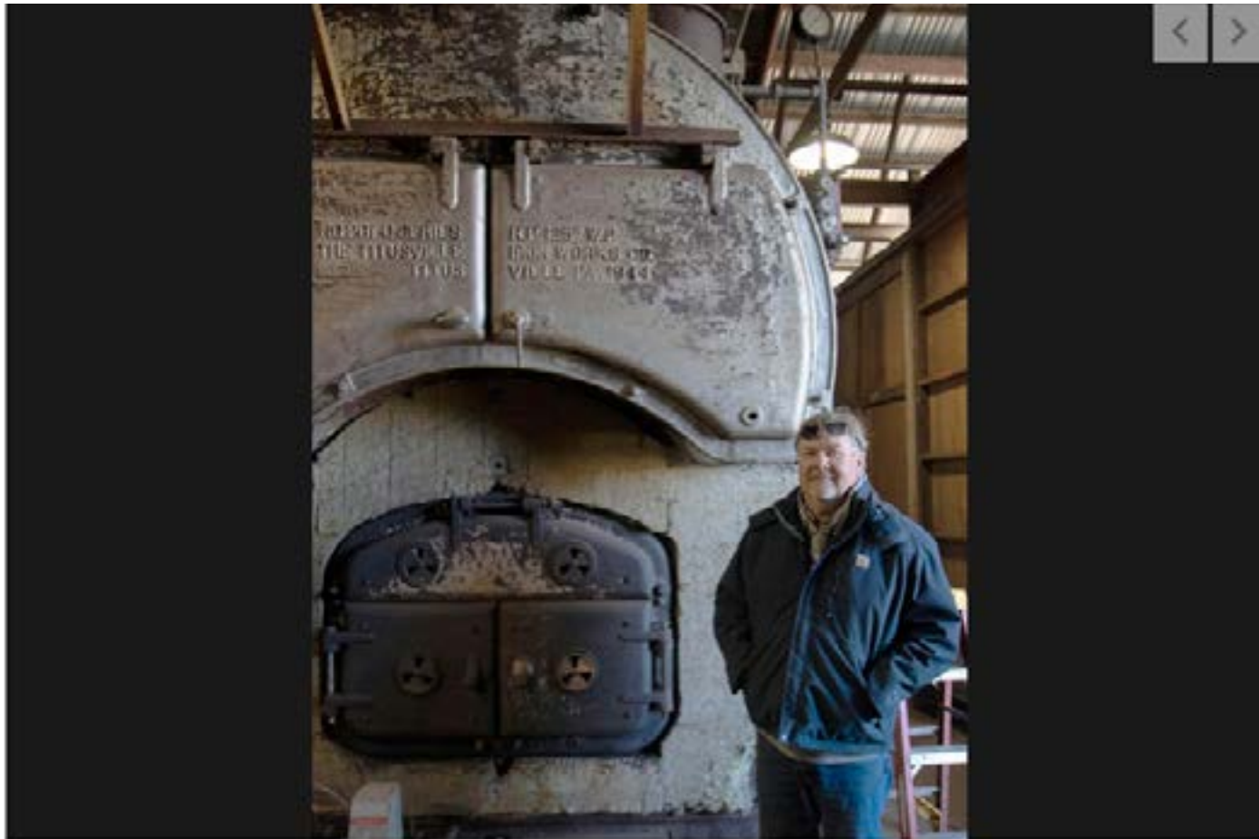
Oregon mint grower John Reerslev stands in his distillery beside a boiler, built in 1944, which he still uses.
